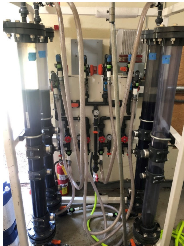
Figure 1: Omni-SORB Oxidation/Filtration Treatment Pilot Assembly.
