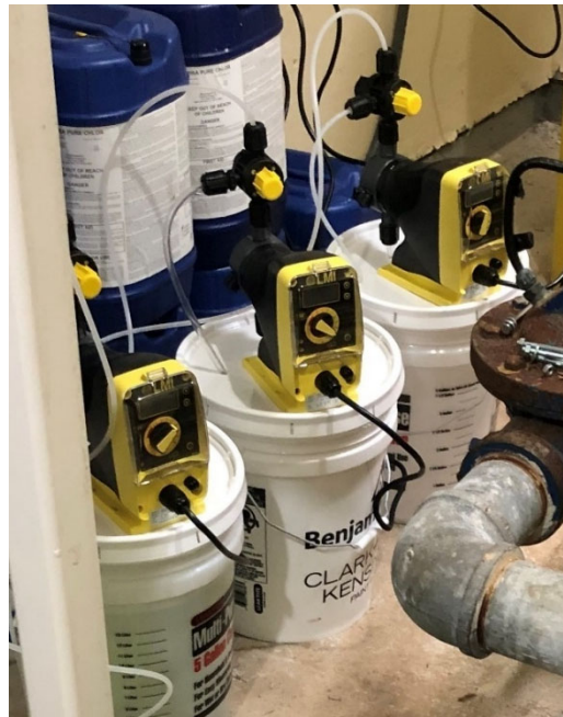
Figure 3: Chemical dosing pumps set up.
