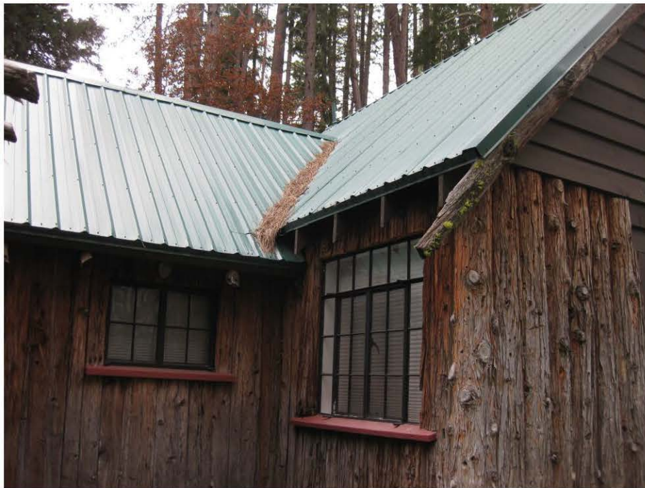
Photo 17-Homes with wood siding are more vulnerable to ignition
