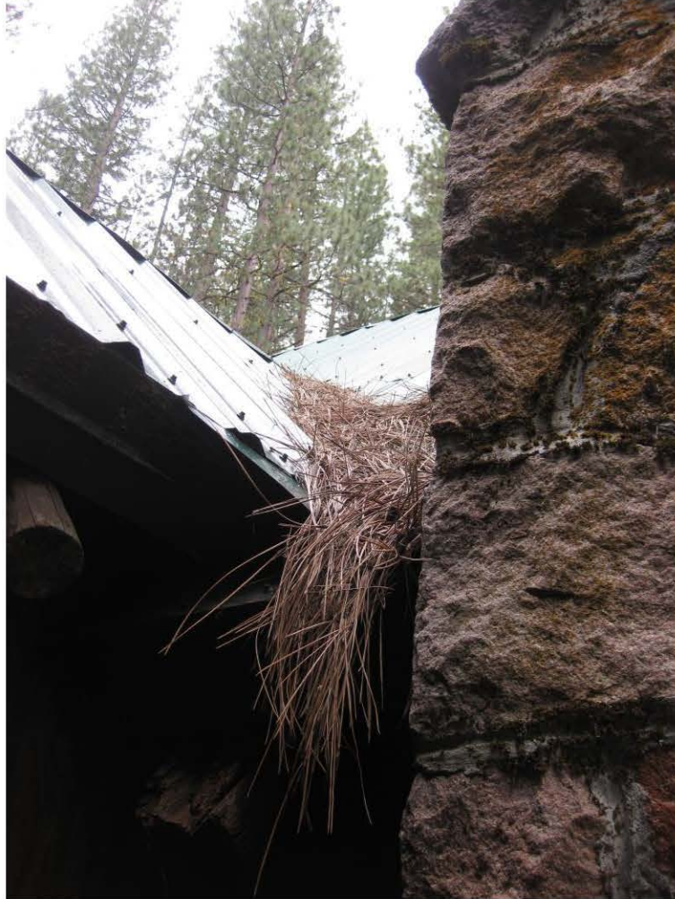
Photo 8-Accumulated debris in the valley of a roof in Plumas Eureka Estates
