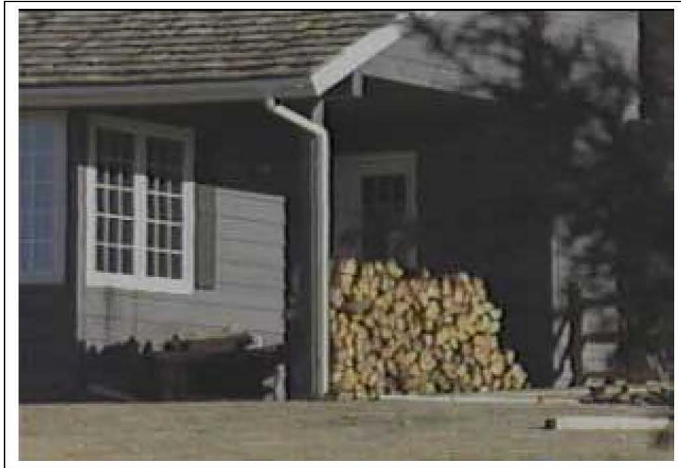
Photograph 12.3. Improper Placement of Firewood
